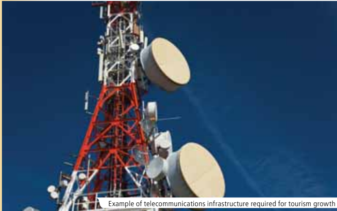
Example of telecommunications infrastructure required for tourism growth
